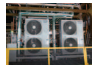
Hamakita Factory's heating system
