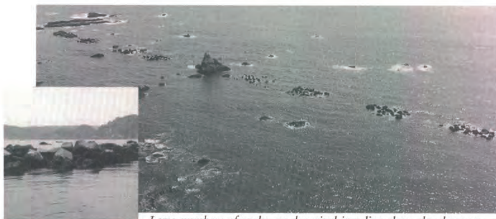
Large numbers of rocks are deposited in a line along the shore to create a breakwall. By breaking wave action, it helps seaweeds grow and creates a favorable place for abalone spat to settle down.
